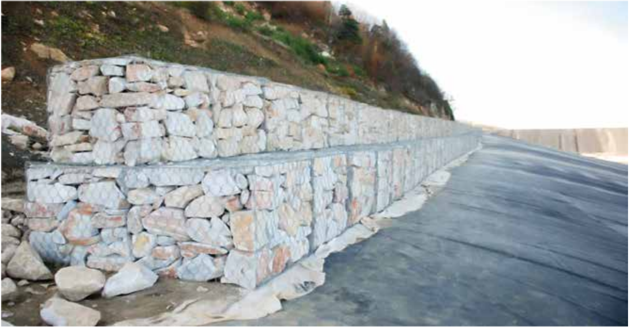
Energy dispersion bank (gabion), which is weaved around the set edge, in order to prevent rock fragments breaking off the slope is indicated in the illustration above.
